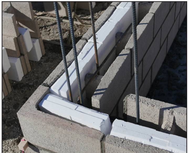
Insulated corners are built using conventional masonry fittings and Hi-R H units
